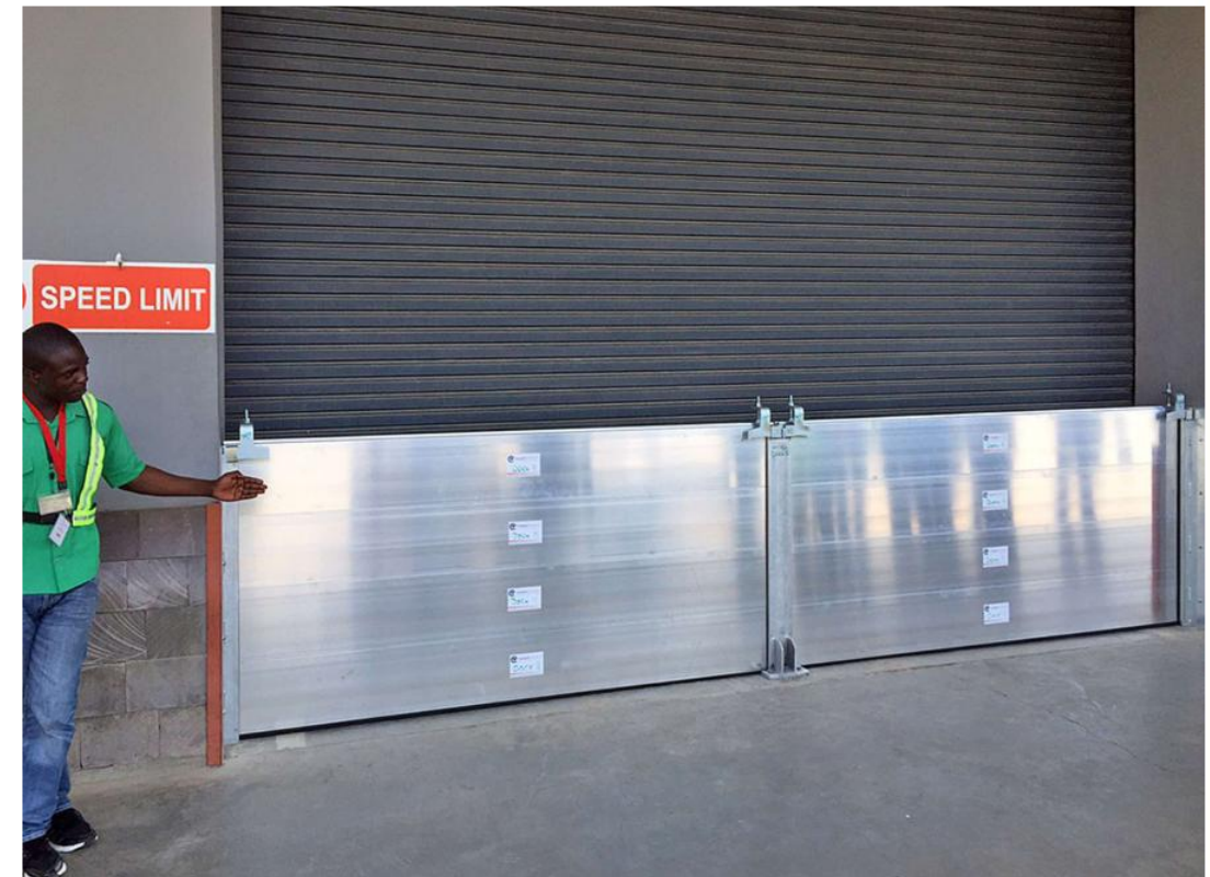
Image: Removable floodwall installed at the Nairobi Airport in Kenya Source: Flood Control International, 2019.
